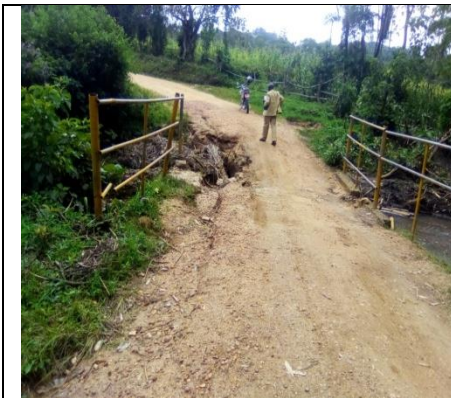
Katete – Kambuga Bridge that drowned after UDN monitors had cautioned the District Engineer, Eng. Eric Mutumba
