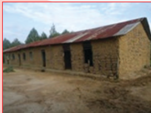
A dilapidated structure at Ntabagwe Primary School, earlier in 2014 and 2015
