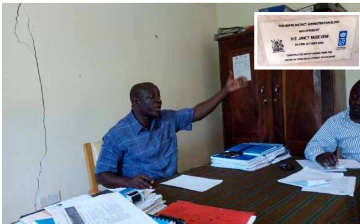
Figure 2: Napak Chief Finance Officer meets Assessment team. Right behind him is a crack that permeates most offices of the Administrative Block built by Central Government less than 5 years before- See Commissioning Plaque inset.
