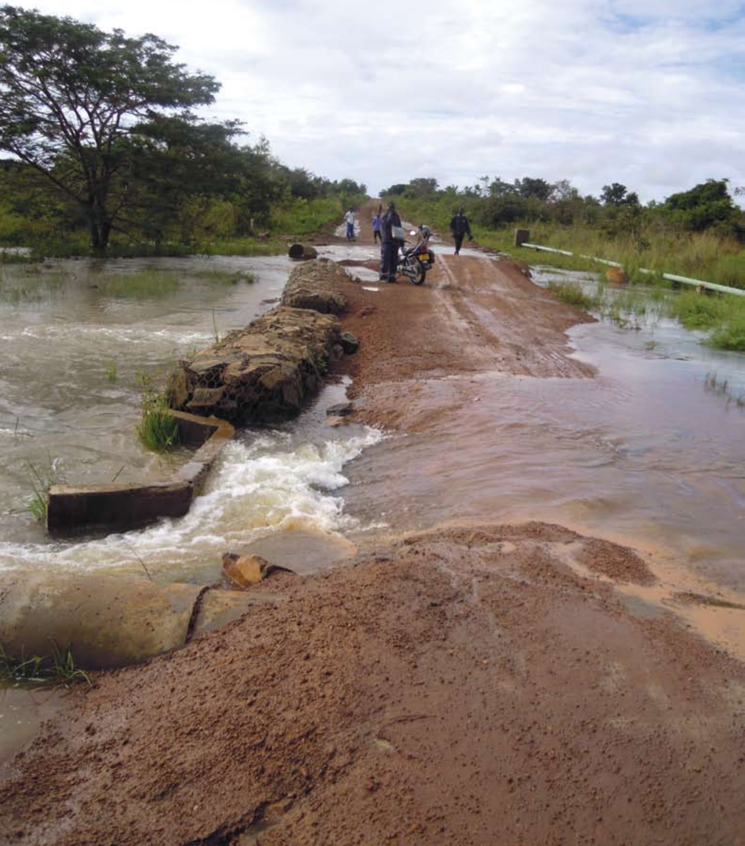
A washed-out bridge on the Amuria-Soroti road.
