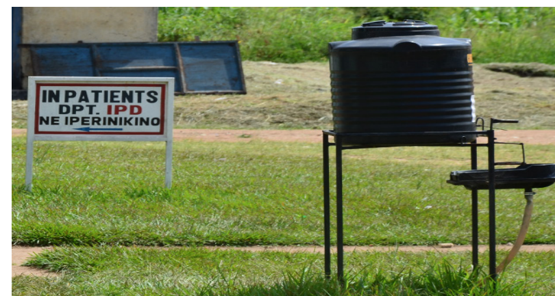
Some of the hand-washing facilities found at Kapelebyong HC IV
