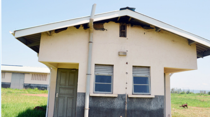
Dilapidated facilities at Bukungu in Buyende district. Locals have shunned the landing site and want an independent audit done on the project by the government
